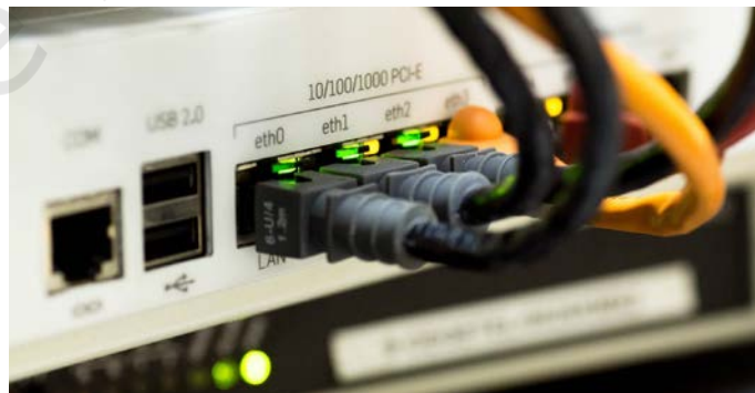
Figure 10.12: Cables connected to a network switch
