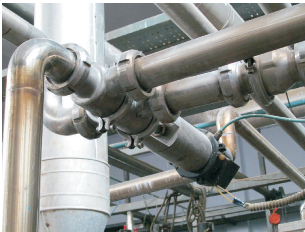
Fig.7.8. Flow diversion valve (FDV)
