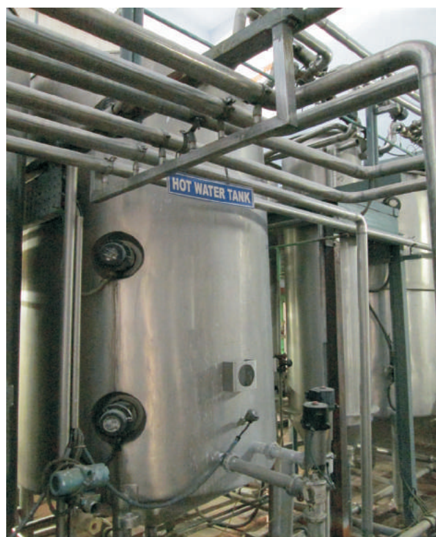
Fig.10.7. Hot water tank
