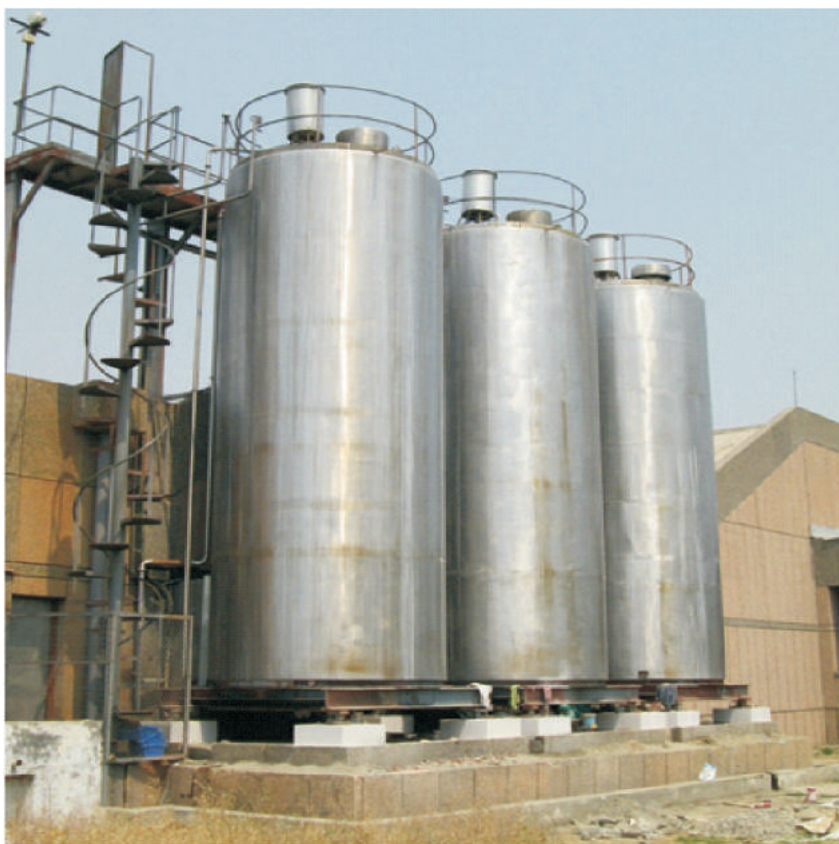
Fig.1.4. Milk storage silos
