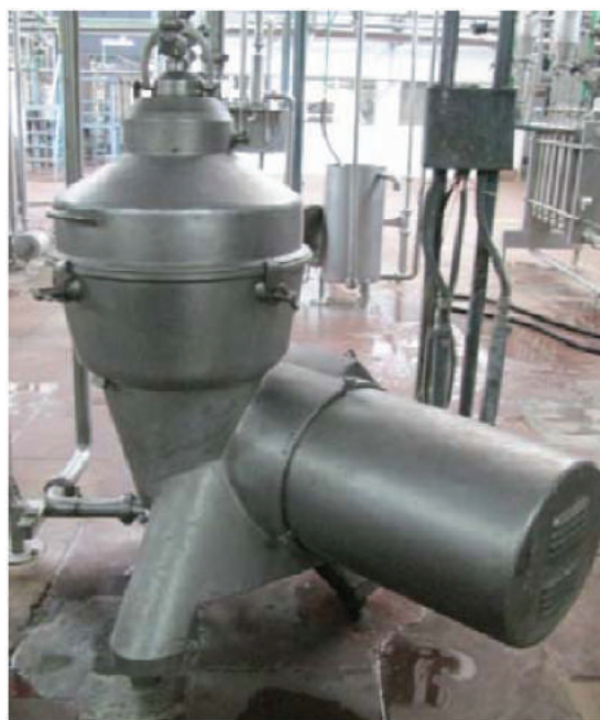
Fig.3.5. In-line modern clarifier
