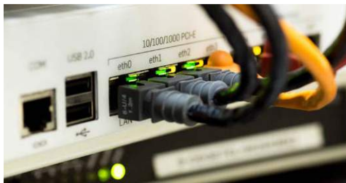
Figure 10.12: Cables connected to a network switch
