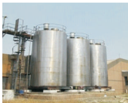
Milk storage tanks
